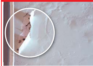
Ceiling is decayed from termite
