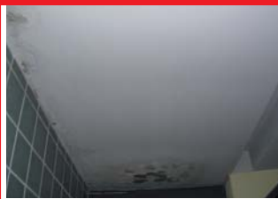
Ceiling is rotted because of water or moisture
